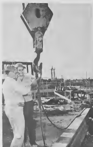
A CRANE is hooked to one end of the bridge's truss section under the supervision of T. O. Lucas, transportation zone foreman. Two cranes lifted the fourteen-ton bridge.
